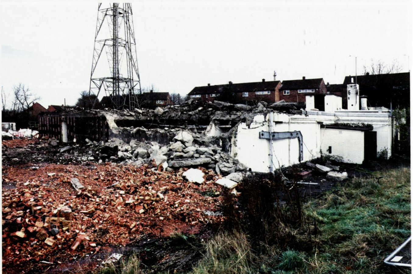
Demolition of the London West AAOR at RAF Uxbridge is underway in November 2012. Photo Paul Francis
